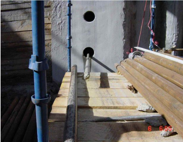
all 508 bores with a measurement tolerance of less than 3 cm at a depth of up to 8 m
